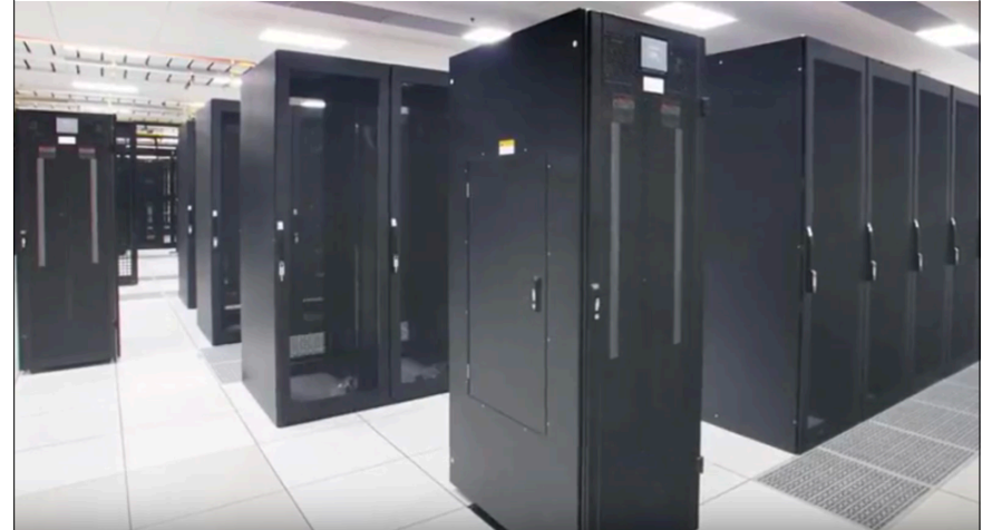
Platz 8: QTS Metro Data Centre , Atlanta USA, with 970,000 sq. ft. of total space one of the largest data centers in the world.
